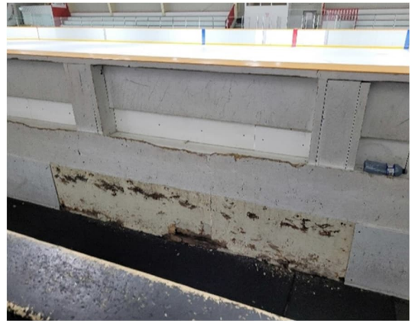
Figure 2-24 Damage to Rink Board in Players Bench Area
