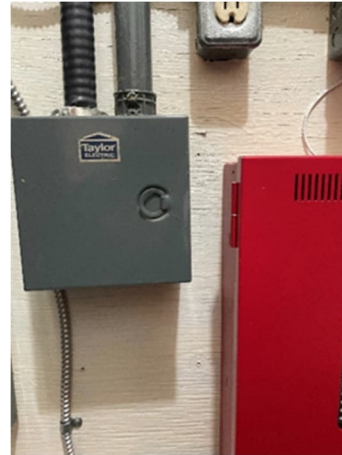
Figure 5-10 High Risk Junction Box (likely replacing the old service connection to the panel in the office)
