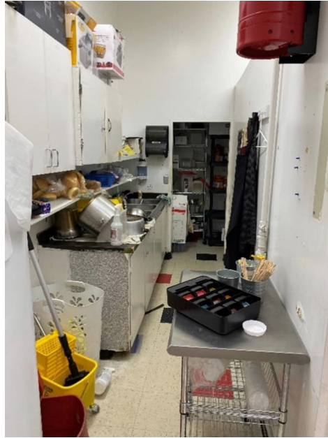
Figure 2-46 Cracked P.Lam Counters & Old Cabinets
