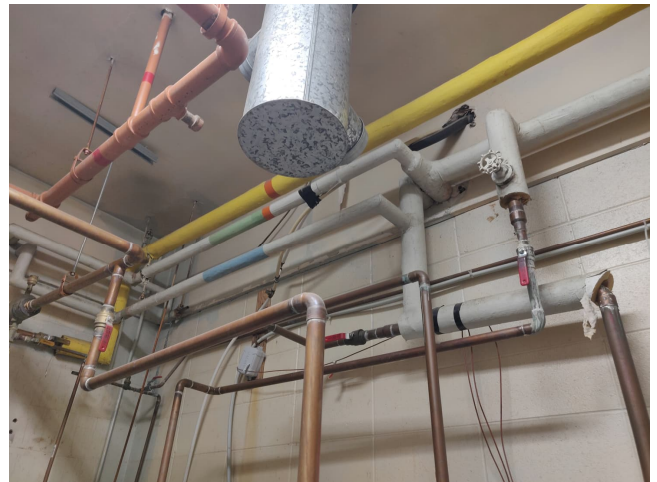
Figure 4-4 Typical Copper Piping in South Mechanical Room
