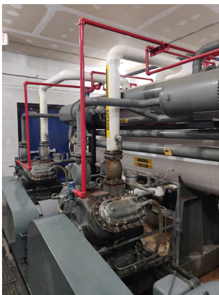
Figure 4-44 Ice Plant Compressors
