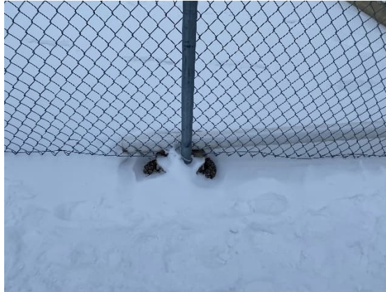
Figure 2-52 Heaving Fence Post
