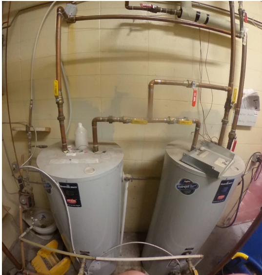
Figure 4-6 Domestic Water Heaters in South Mechanical Room
