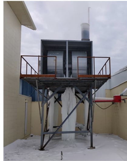
Figure 4-47 Ice Plant Condensing Unit
