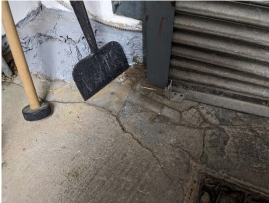
Figure 3-24 Cracking in Southwest Corner of Zamboni Room
