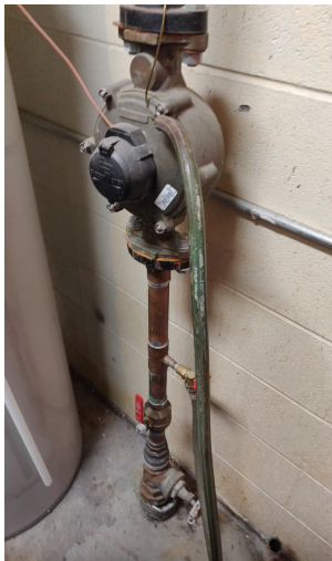
Figure 4-3 Domestic Water Service Entry in South Mechanical Room
