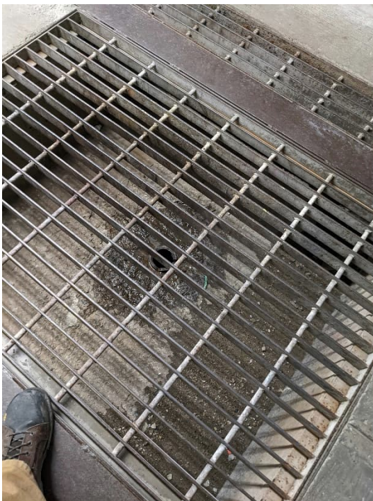
Figure 3-26 Extreme Concrete Degradation in Zamboni Room West Pit
