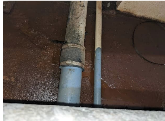
Figure 3-25 Moisture and Discoloration in Base of Zamboni Room East Pit
