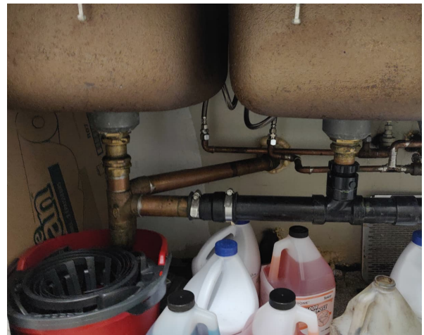
Figure 4-2 Exposed Copper and PVC Sanitary Piping Under Concession Sink
