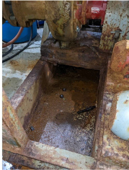
Figure 3-29 Corrosion on Equipment, Supports and Skid
