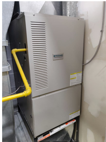
Figure 4-40 Furnace Serving Change Room Addition
