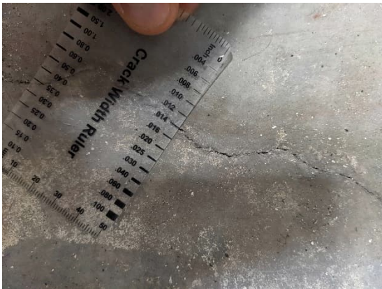
Figure 3-20 Cracking in Mechanical Room
