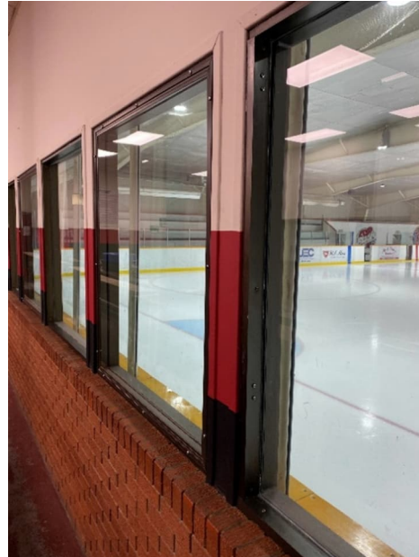
Figure 2-38 Windows Are Not Code Compliant
