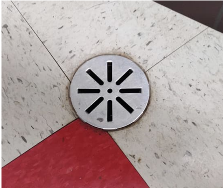
Figure 4-12 Typical Floor Drain in Original Building Area
