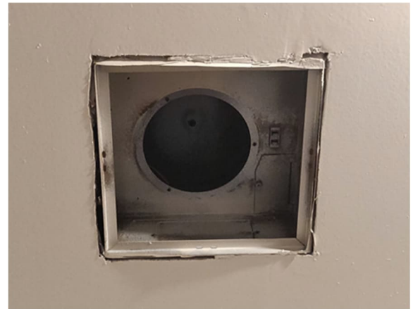
Figure 4-39 Typical Cabinet Exhaust Fan Missing Grille
