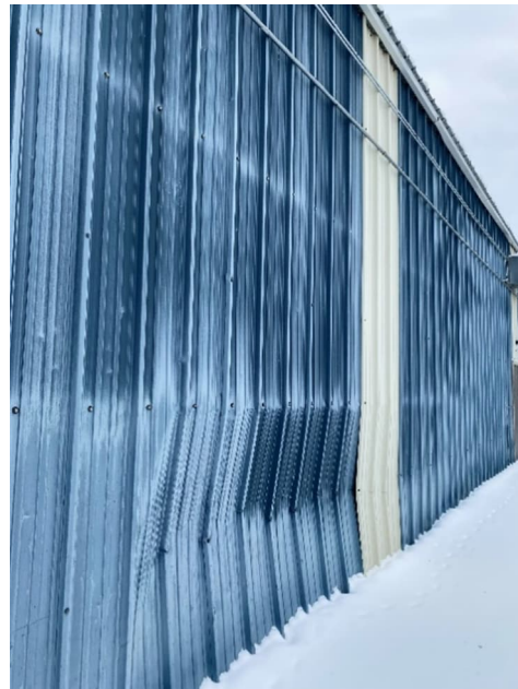
Figure 2-10 Damaged Exterior Cladding
