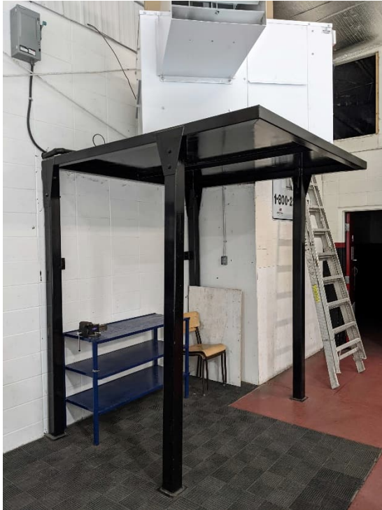
Figure 3-44 Southeast Dehumidifier Steel Frame
