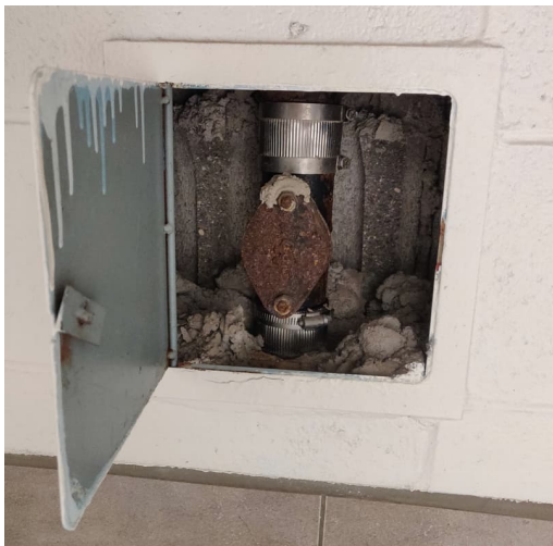
Figure 4-1 Typical Cast Iron Sanitary Riser
