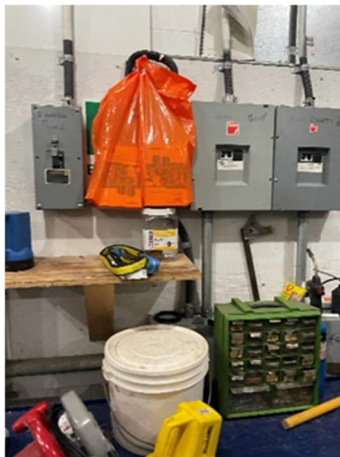
Figure 5-7 Gutter to Breakers (feeds the Bleacher Panel, Lobby Electrical Room and Office (Original))
