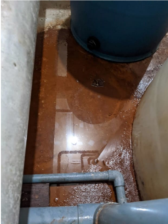
Figure 3-22 Ponding of Water Near Brine Tank in Ice Plant
