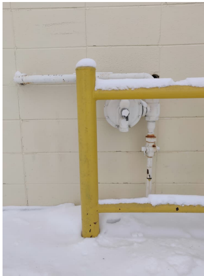
Figure 4-24 Building Gas Regulator
