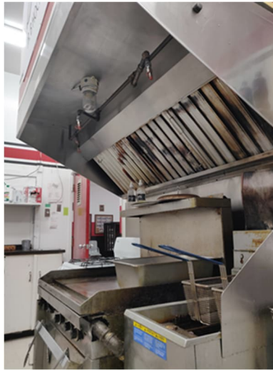
Figure 4-53 Range Hood with Fire Suppression System
