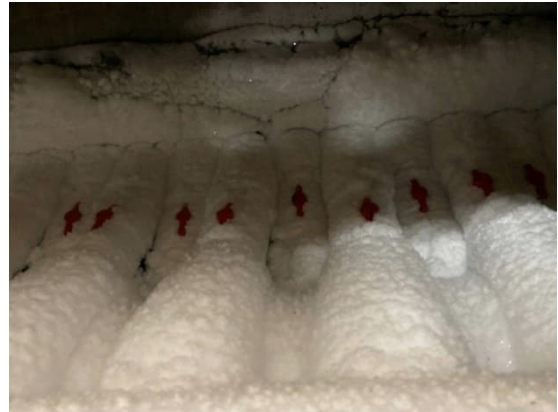
Figure 2-20 Frosted Pipes in Header Trench
