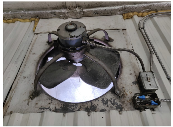
Figure 4-29 Typical Arena Exhaust Fan
