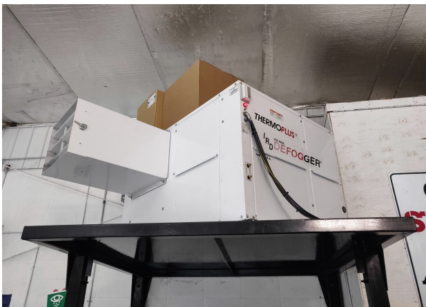
Figure 4-30 Typical Dehumidifier in Arena
