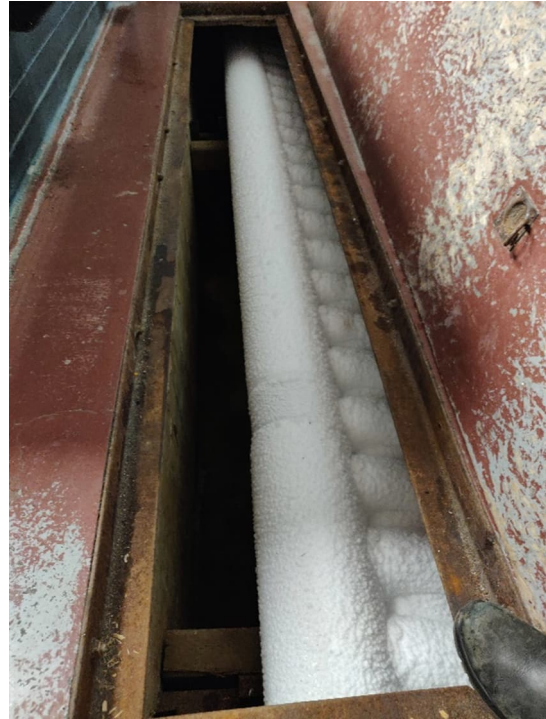
Figure 3-11 Header Trench Shelf Angle Corrosion
