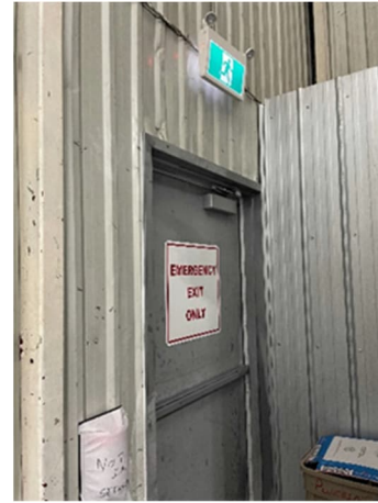
Figure 5-21 Modernized Emergency Light - Battery Combo
