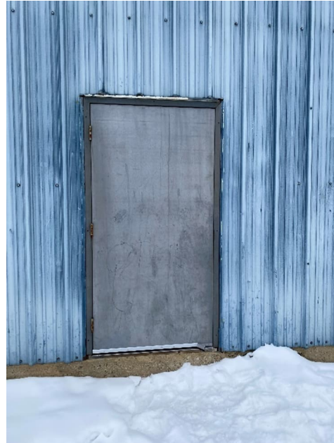
Figure 2-37 Unpainted Exit Door &amp; Threshold Damaged
