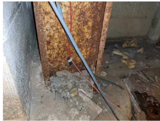
Figure 3-43 Corroding Pre-Engineered Steel Column Near Brine Tank
