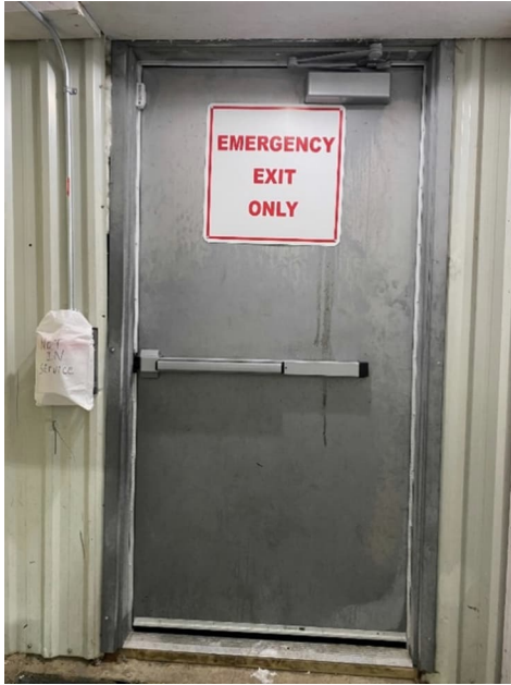
Figure 2-36 Frosting on Exit Door
