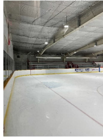
Figure 5-19 Arena LED Lighting Without Mechanical Protection (Def)
