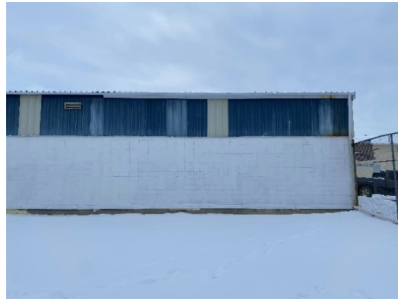
Figure 2-12 Rust Visible on Southwest Corner
