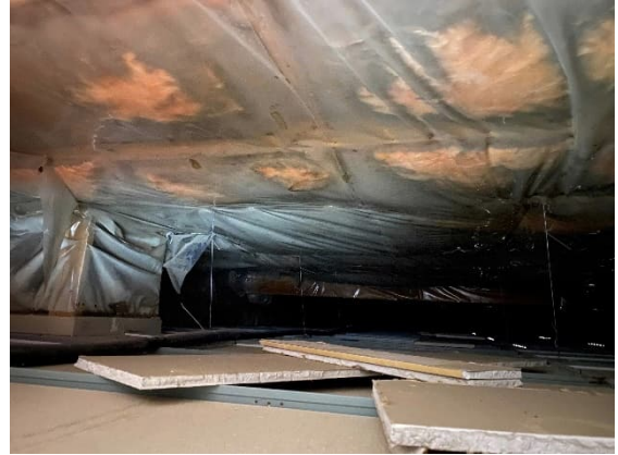
Figure 2-16 Water Damaged Fiberglass Insulation
