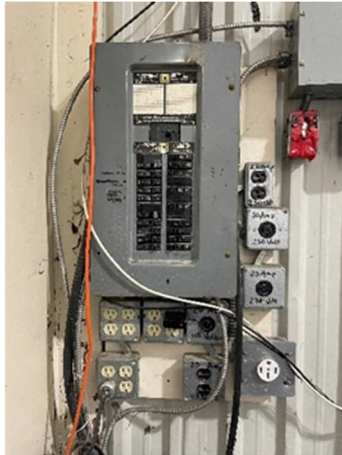
Figure 5-9 Bleacher Power Panel (accessible to public)
