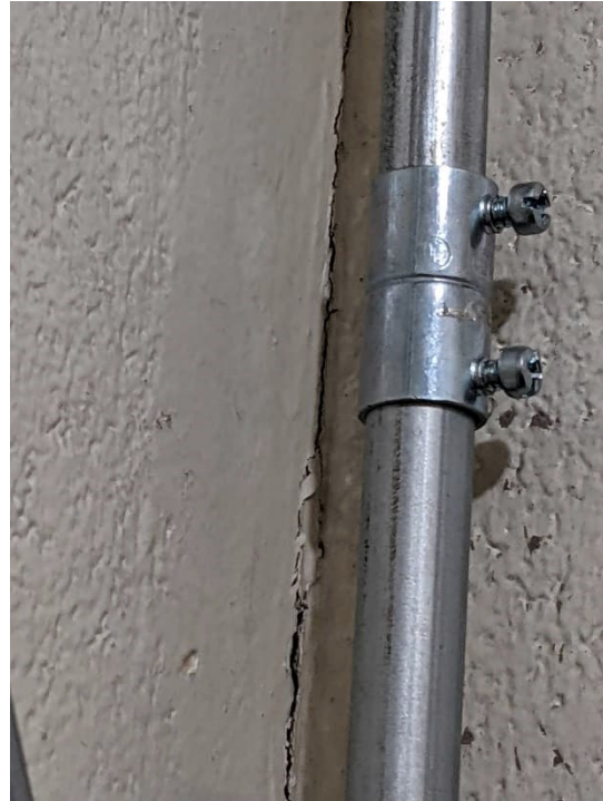
Figure 3-7 Cracking of 0.60 mm in Janitor Closet
