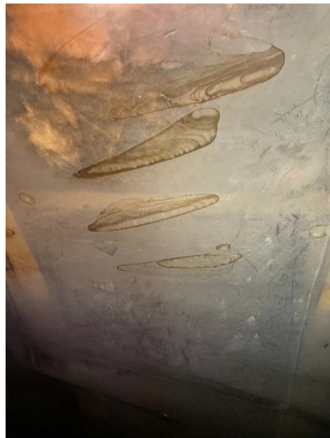
Figure 2-14 Water Stains on Fiberglass Insulation
