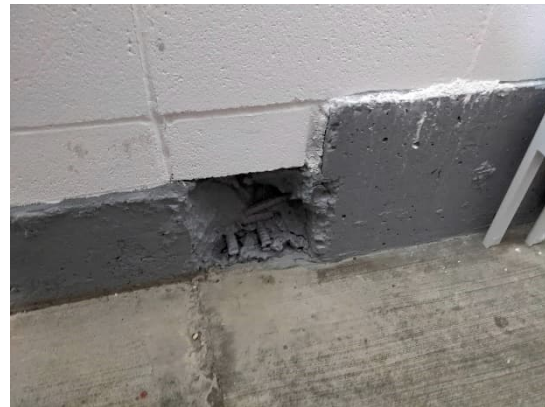
Figure 3-17 Irregular/Poor Transition in Zamboni Room Wall
