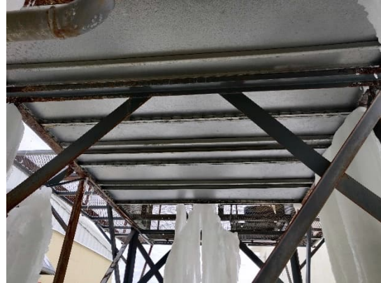
Figure 3-47 Condensing Unit Steel Frame Corrosion and Ice
