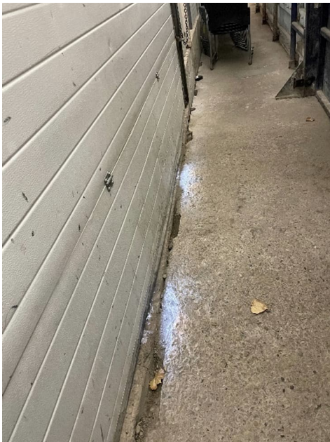
Figure 2-21 Concrete at Overhead Door Requires Patching
