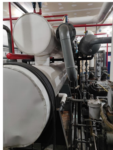
Figure 4-45 Ice Plant Chiller
