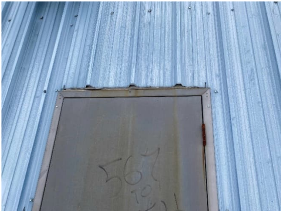
Figure 2-11 No Flashing Over Exit Door
