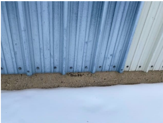
Figure 2-7 No Base Flashing
