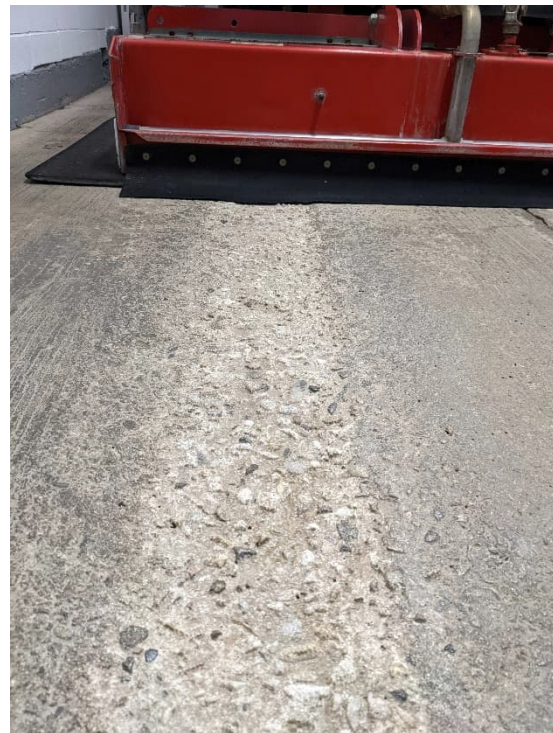
Figure 3-27 General Slab Wear from Ice Resurfacer Traffic
