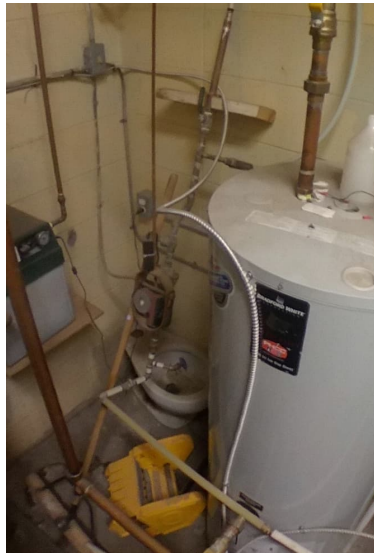
Figure 4-5 Haphazard Domestic Water Piping in Mechanical Room
