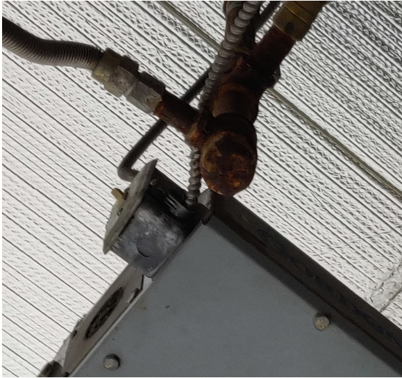
Figure 4-26 Typical Corroded Gas Pipe Fitting in Arena
