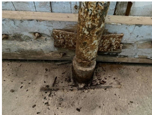
Figure 2-25 Rusting on Metal Support for Dasher Board
