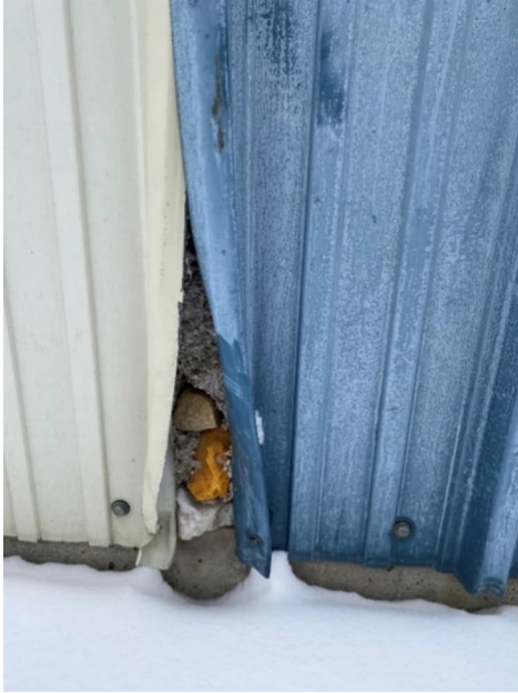
Figure 2-9 Damaged Exterior Cladding
