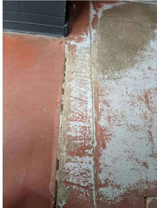
Figure 3-9 Debonding of Bond Break at Beam Line Between Rink and Lobby
