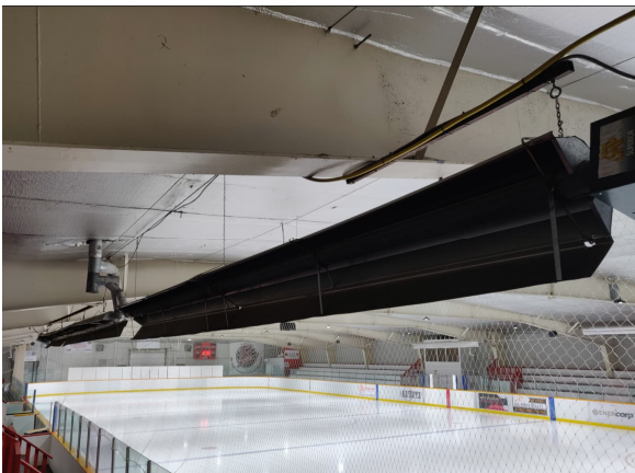
Figure 4-28 Typical Tube Heaters in Arena
