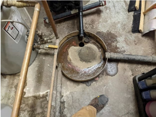
Figure 3-10 Deterioration of Concrete in Front Mechanical Room
