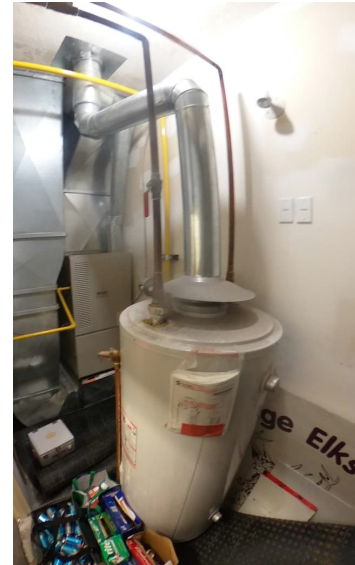
Figure 4-7 Water Heater in 2010 Expansion Area
