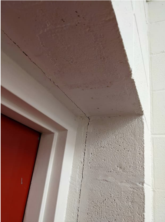
Figure 3-6 Cracking of up to 1.5 mm in Size at Curling Rink Walkway Access Door
