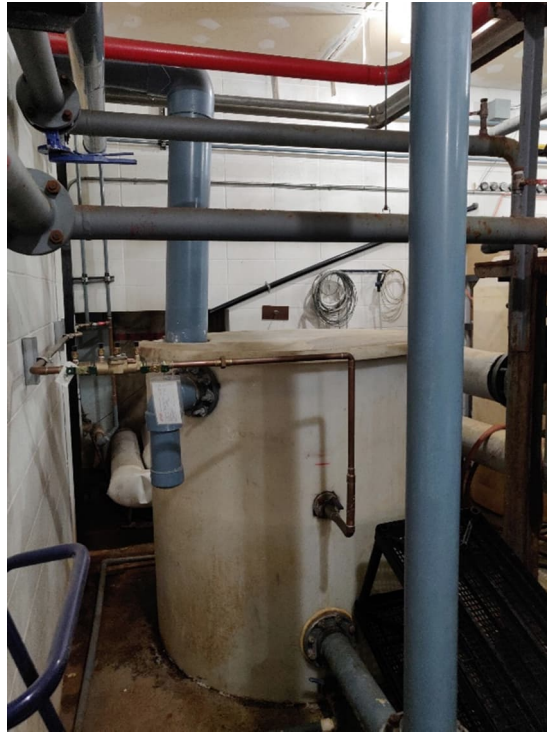
Figure 3-30 Brine Tank in Southwest Corner of Ice Plant
