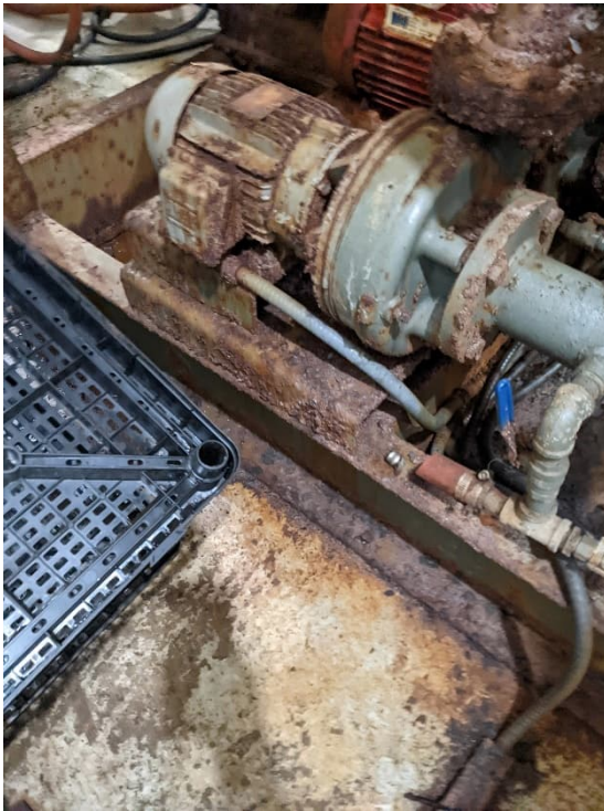
Figure 3-28 Corrosion on Equipment, Supports and Skid
