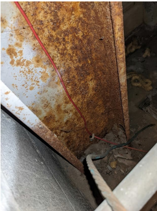
Figure 3-42 Corroding Pre-Engineered Steel Column Near Brine Tank
