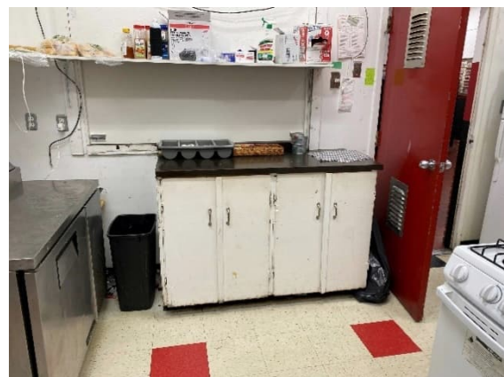
Figure 2-45 Old & Damaged Millwork
