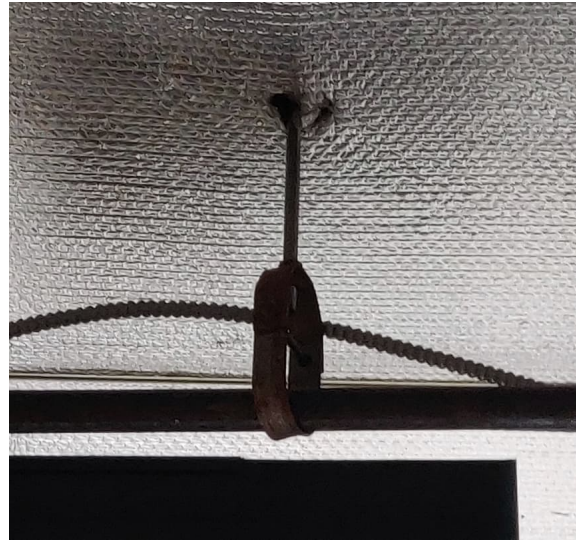
Figure 4-27 Typical Corroded Gas Pipe Hanger in Arena
