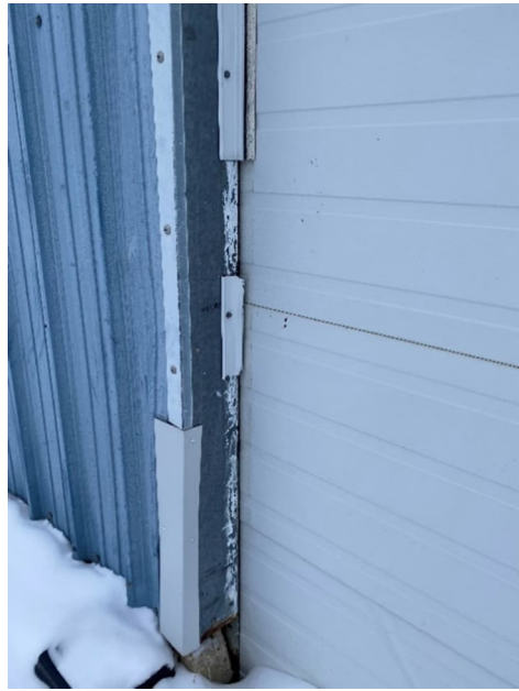
Figure 2-31 Damaged Seals on Overhead Door
