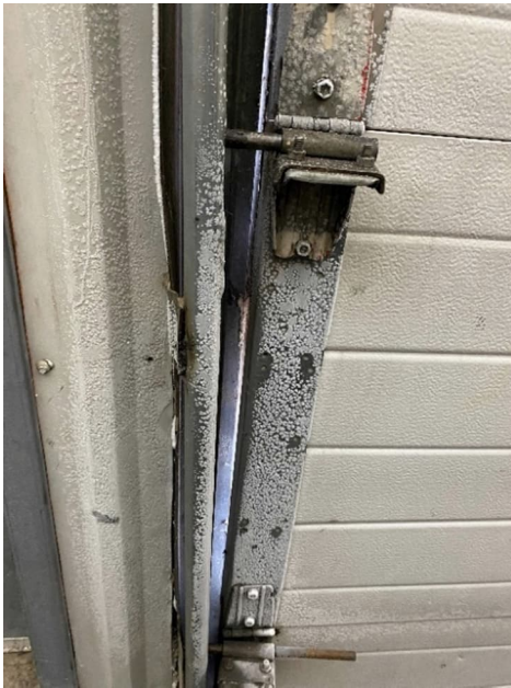
Figure 2-30 Frosting on Overhead Door
