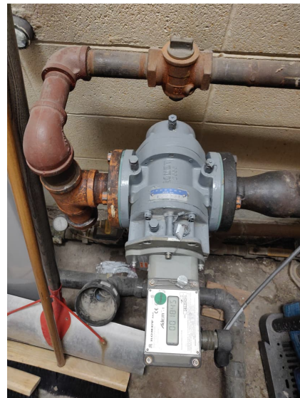
Figure 4-25 Building Gas meter
