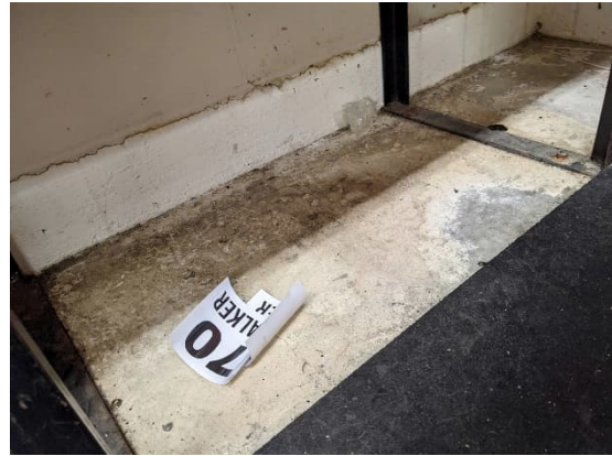
Figure 3-15 Cracking at Bottom of Masonry Wall and Curb in Dressing Room 5
