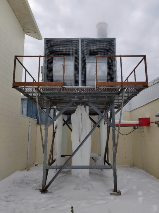
Figure 3-46 Exterior Condensing Unit Steel Frame
