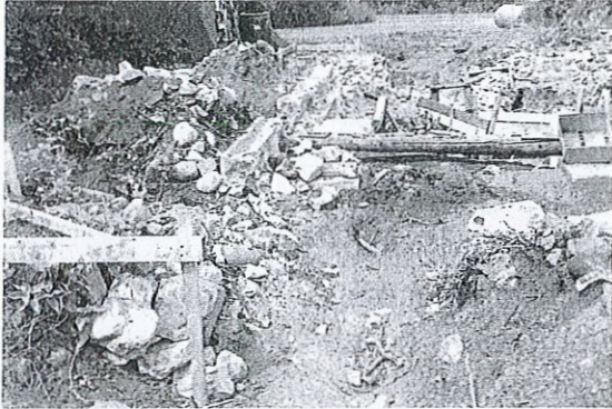
Debris under the house
